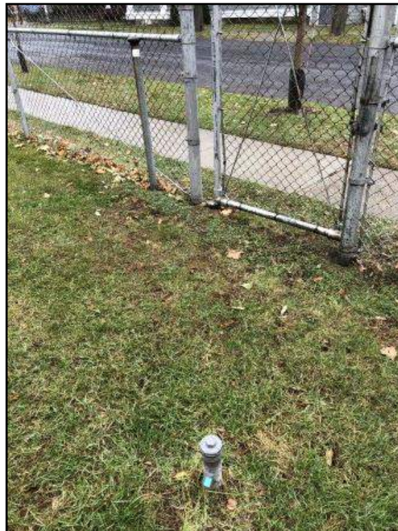
Fill port (bottom, center) and vent (top, left of center) for 1,000-gallon heating oil UST, NE corner of building exterior, facing NE
