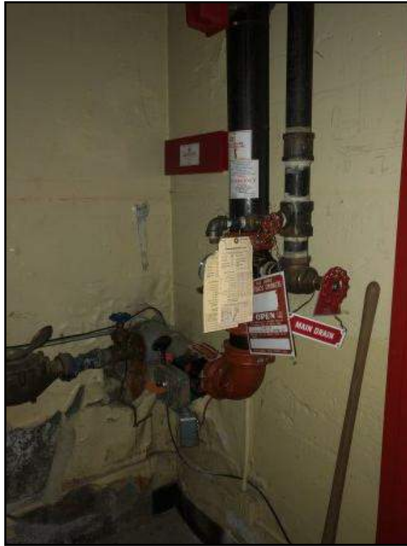
Village of Rhinebeck water supply connection
