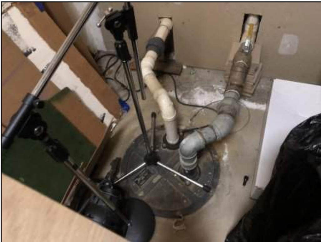
Sump or possible pump in basement to septic system
