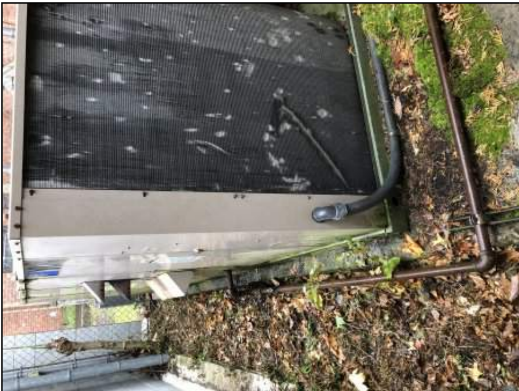
Propane lines to air handlers
