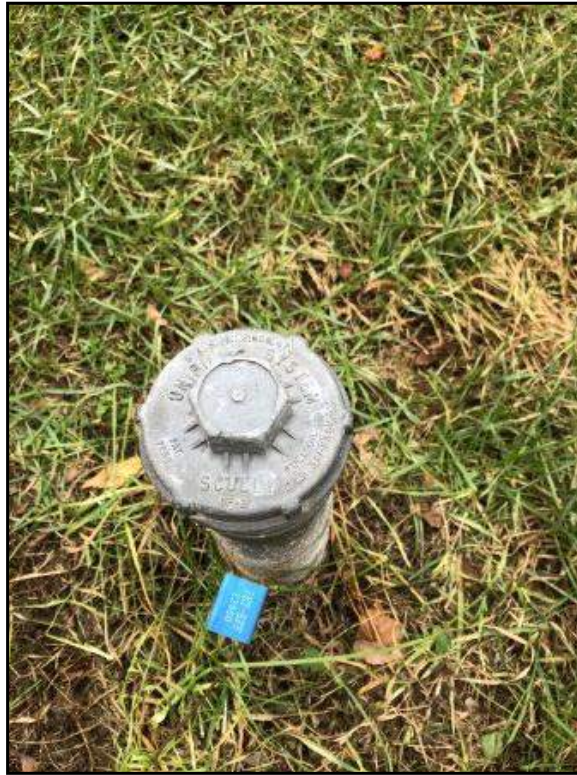
1,000-gallon UST fill port
