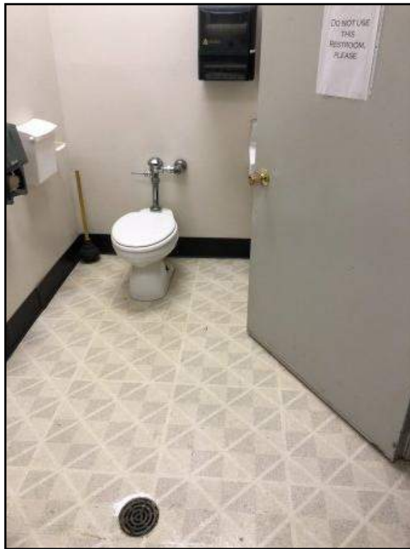
Floor drain in bathroom (2)
