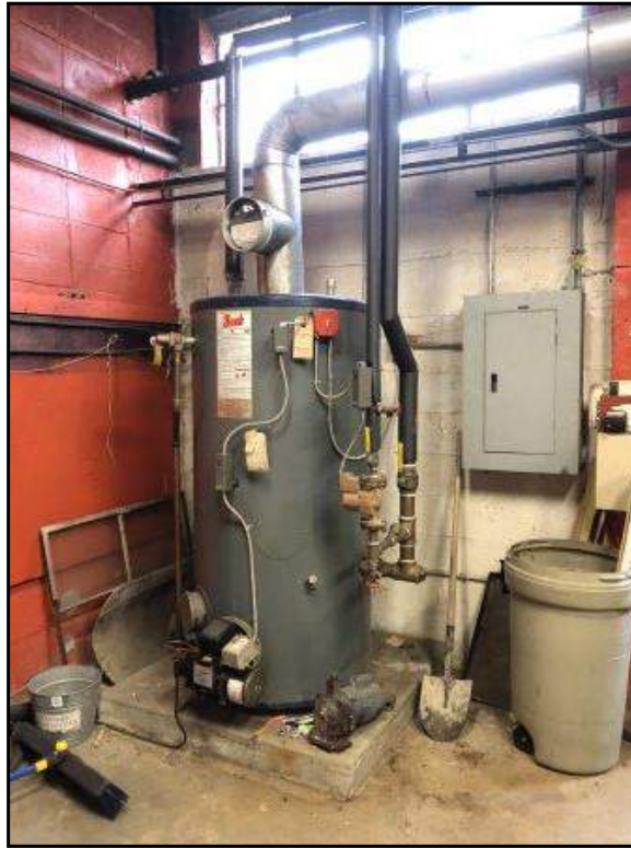
Hot water tank in boiler room
