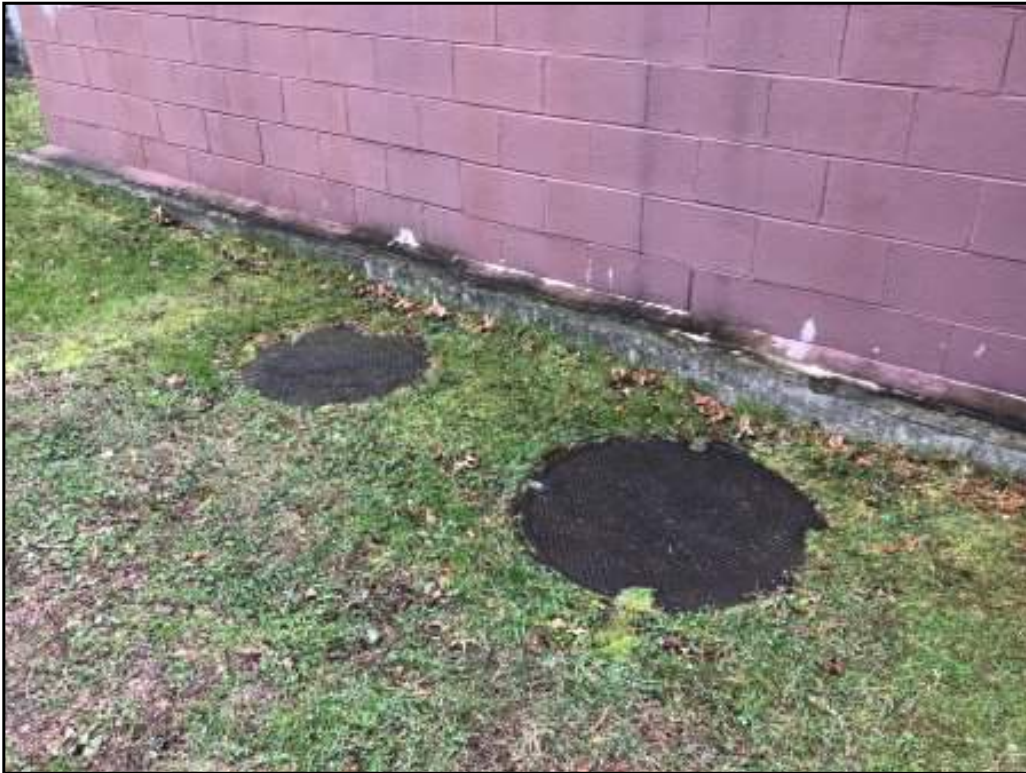
Septic tank covers
