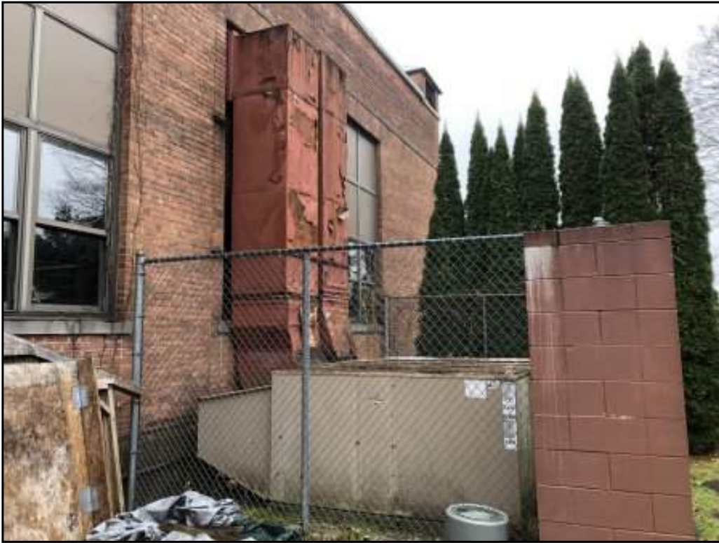
Air handlers for AC at northern side of building
