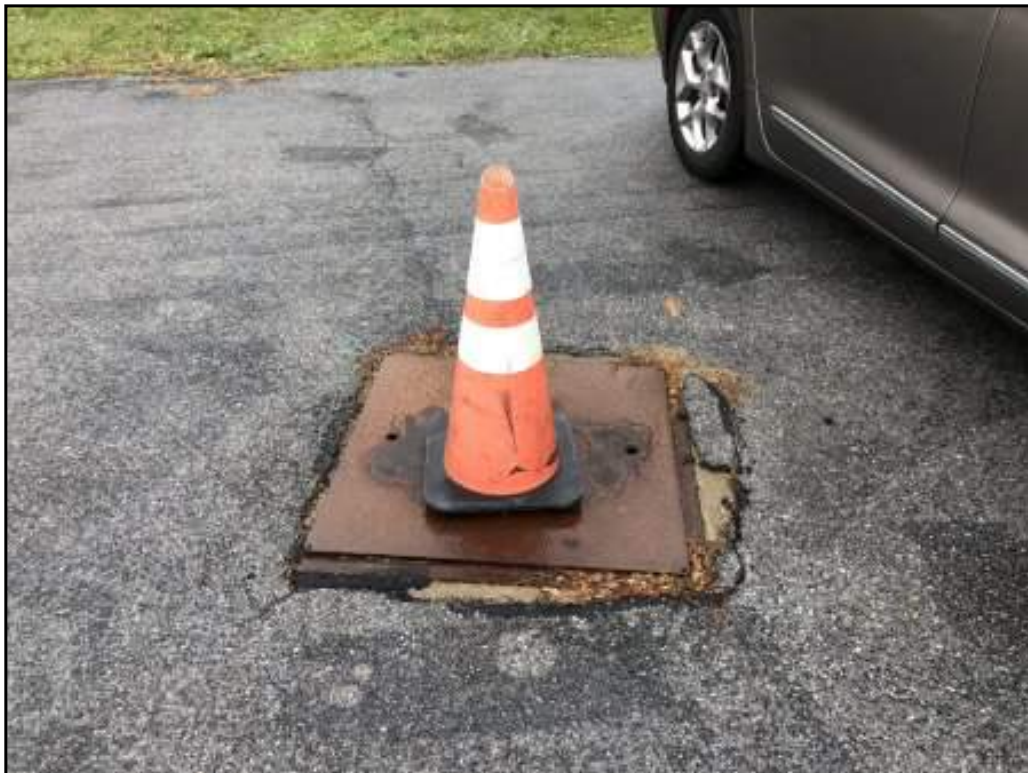
Metal plate cover over likely septic tank in parking lot
