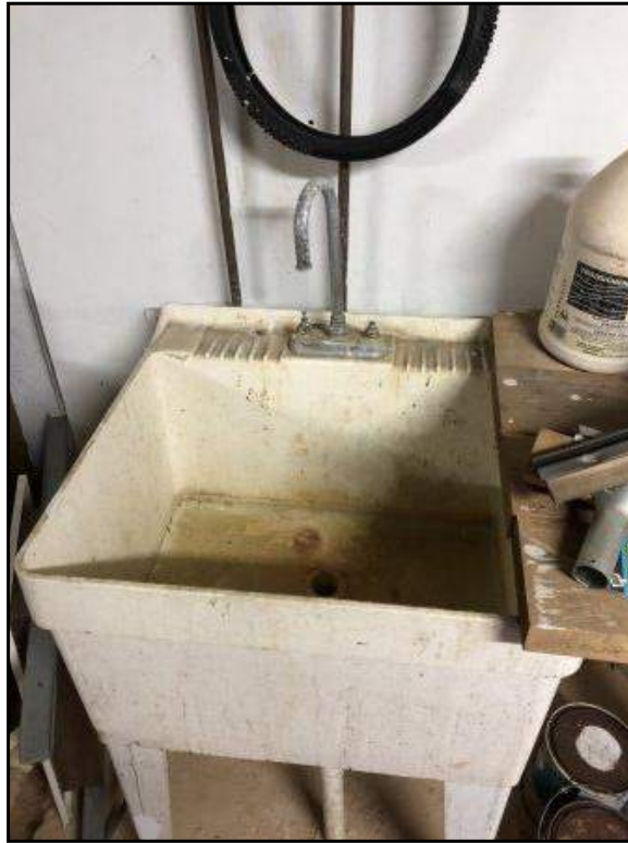
Slop sink in basement
