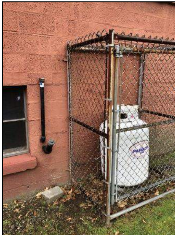
120-gallon propane tank on eastern side of building
