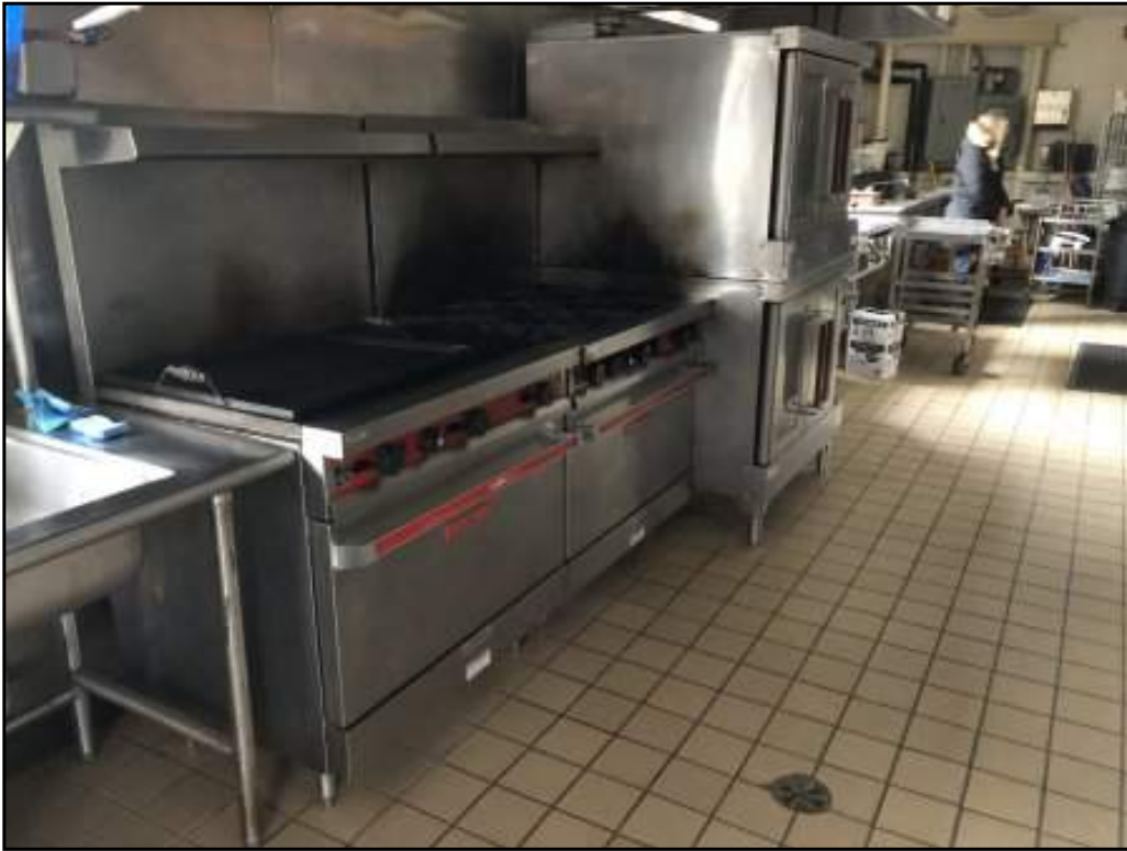
Floor drain in commercial kitchen (1)
