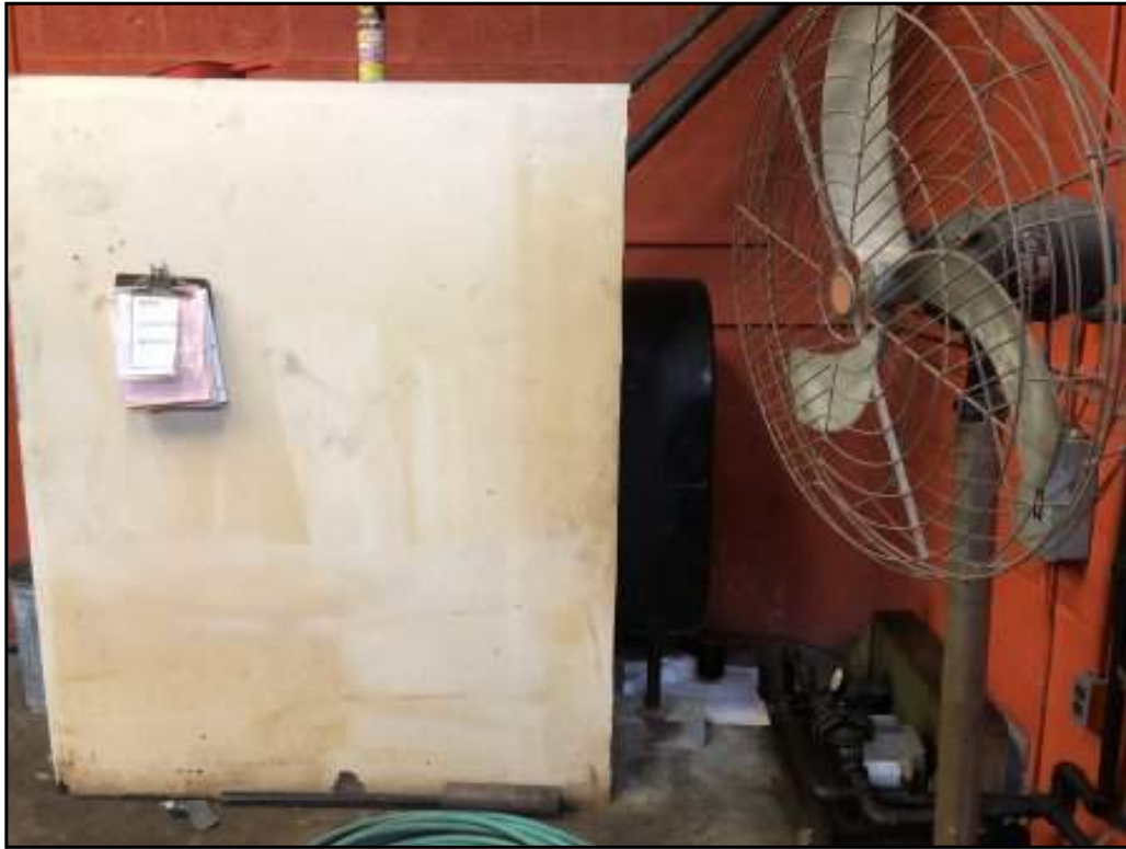
Partial enclosure for 275-gallon AST in boiler room
