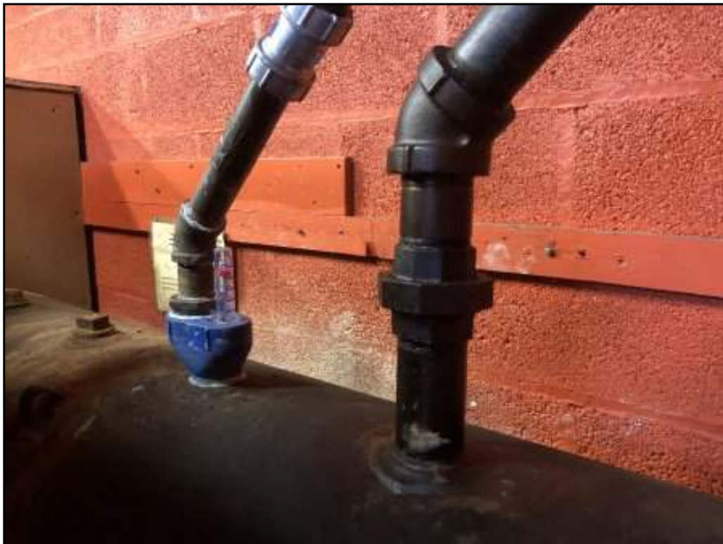
275-gallon AST in boiler room
