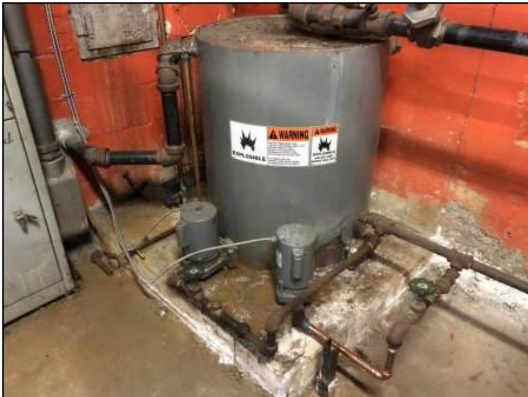
Hot water or steam tank in boiler room
