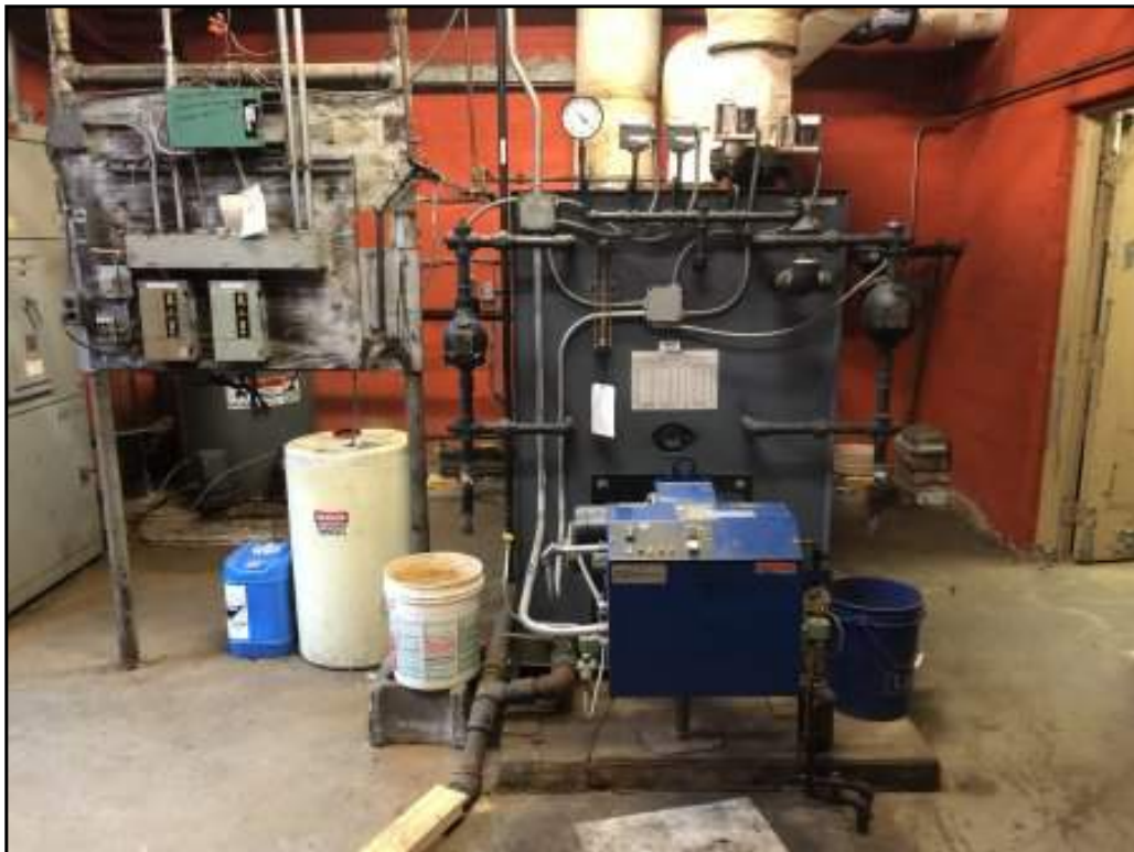
Steam boiler in boiler room
