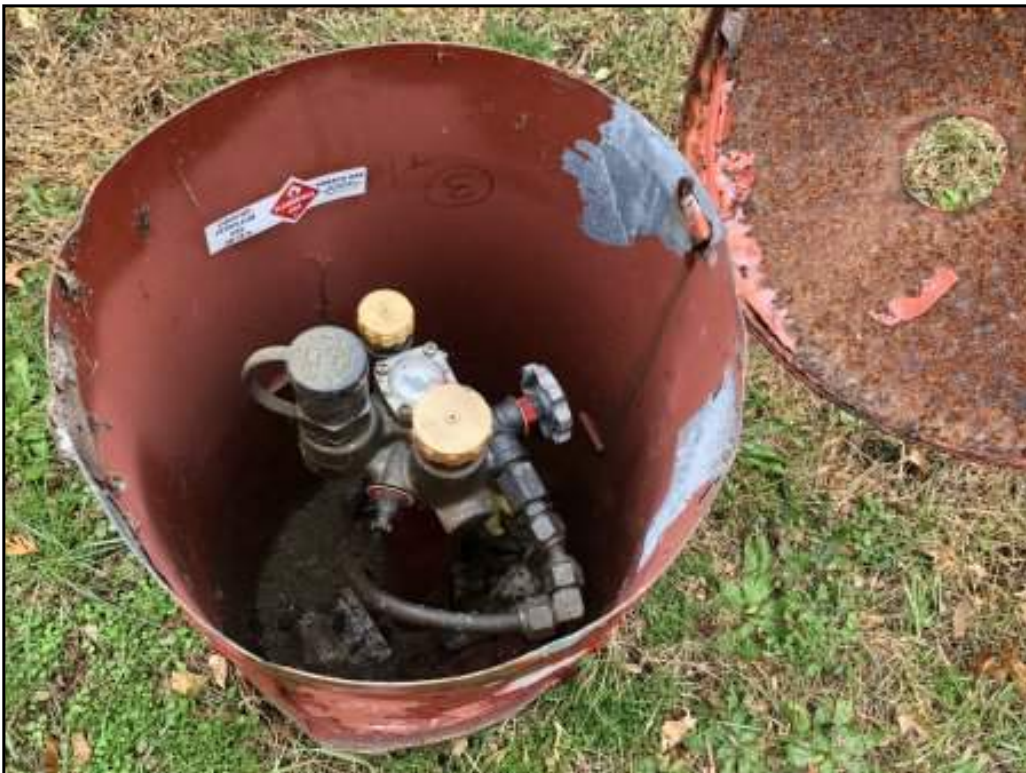
Access to buried propane tanks
