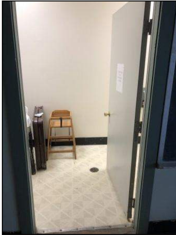
Floor drain in bathroom (1)
