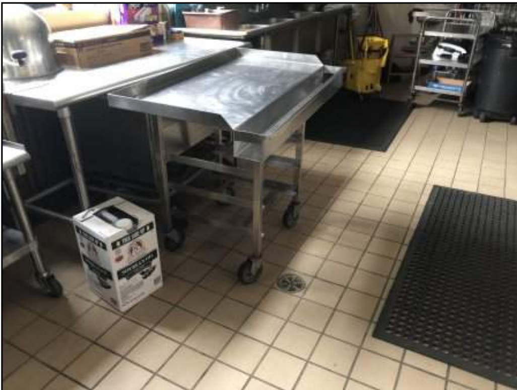
Floor drain in commercial kitchen (2)
