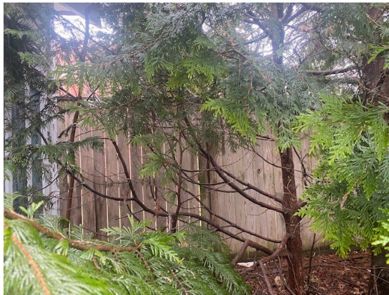
Figure 2. A portion of the privacy fence running along the southern boundary of the Haak & Chumas property, the installation of which had been mandated by the Village ZBA.
